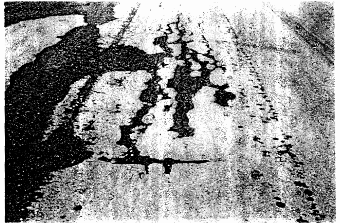
FIG. X1.2 Low-Severity Alligator Cracking
