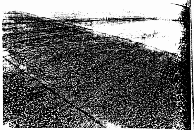
FIG. X1.8 Medium-Severity Alligator Cracking, Approaching High Severity (Example 2)
