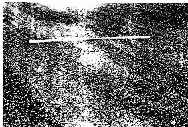
FIG. X1.7 Medium-Severity Alligator Cracking, Approaching High Severity (Example 1)
