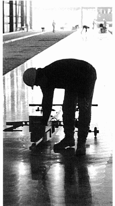
Xorex™ Steel Fiber Reinforced Concrete has been used to achieve many superflat ( F_{min} -100) floors.
