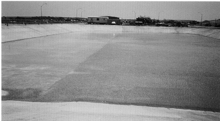
Xorex™ Steel Fiber was the only reinforcement in this water retention pond in Queensland, Australia.
