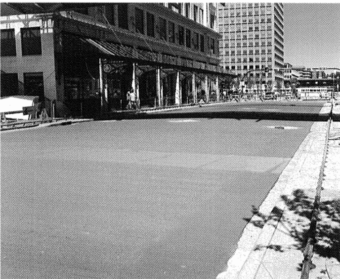
Calgary, Alberta, Canada - City street overlaid with 4" of Xorex™ Steel Fiber Reinforced Concrete.
