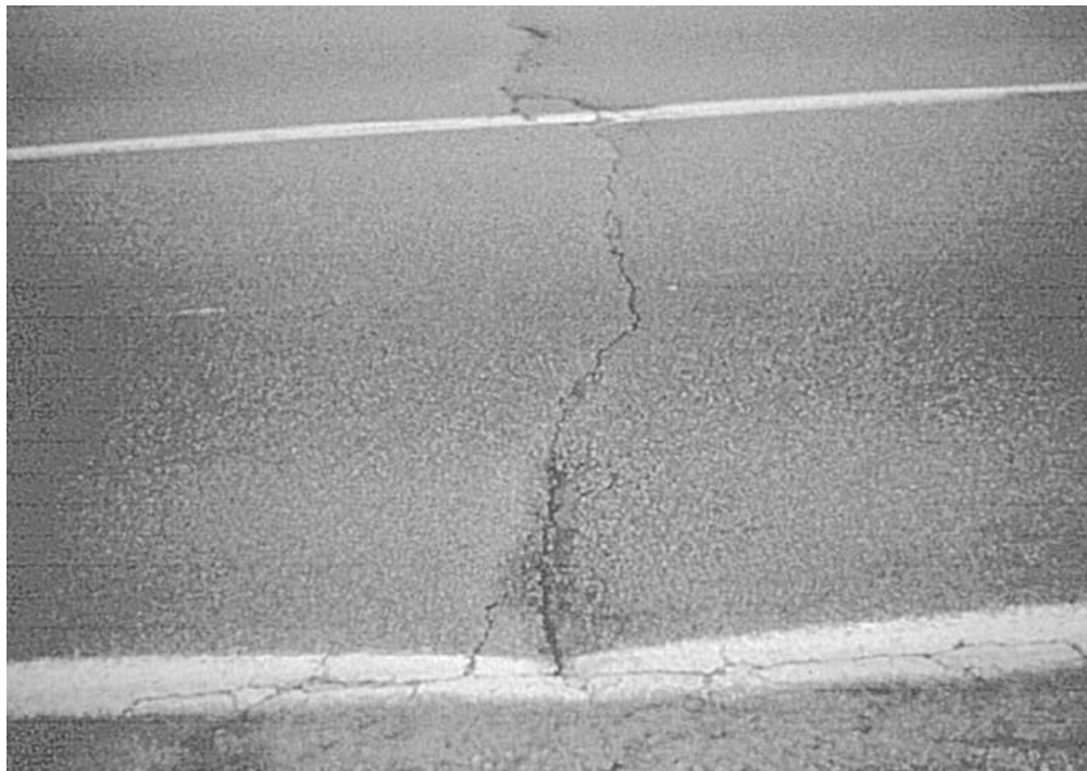
Figure 2-1.12. Surface distress of HMA pavement surface layer with underlying stripping problem.
