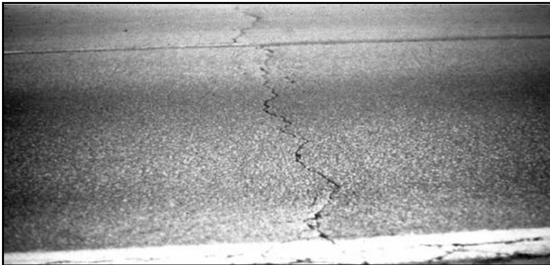
Figure 2-1.9. Medium severity transverse crack in HMA surface.
