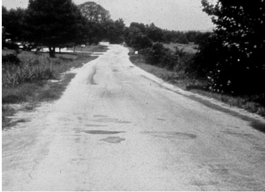
Figure 2-1.13. Example of heavily oxidized HMA surface layer.
