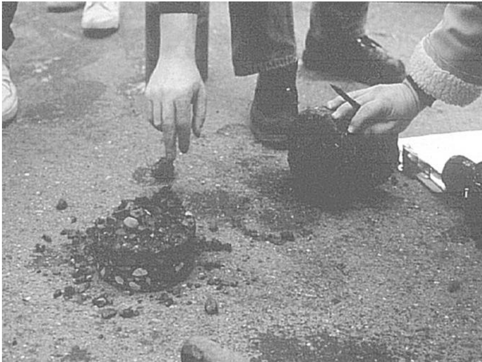
Figure 2-1.11. Example of “stripped” HMA layer.
