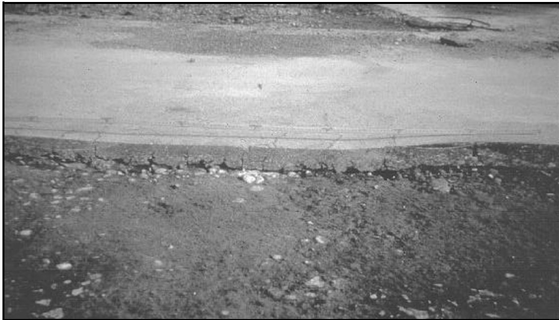
Figure 2-1.4. AASHO road test section exhibiting fatigue and frost heave damage.
