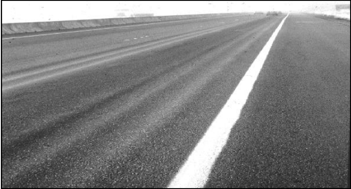
Figure 2-1.8. Example of HMA surface exhibiting double ruts in each wheelpath.
