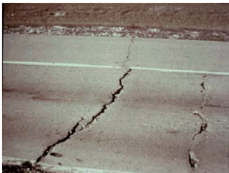
Transverse Crack - High Severity
