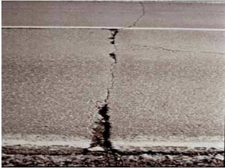
Transverse Crack - High Severity
