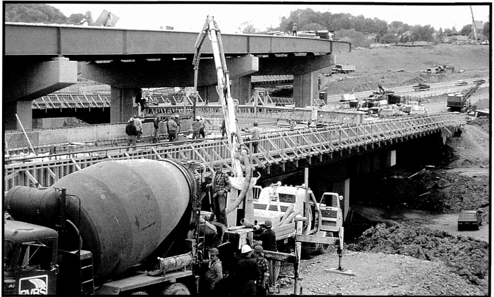
The C-450 on this bridge deck is equipped with two power transition adjustors (PTA) for on-the-go crown elevation changes which are installed at pin-connected points.
