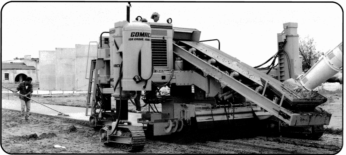
Simultaneous fine grade trimming and slipforming a 10 ft. (3.05 m) wide sidewalk, 4 in. (102 mm) thick is an application for the COMMANDER III. This contractor utilizes the versatility of the COMMANDER III by switching from sidewalk to curb and gutter and also pre-trimming projects.
