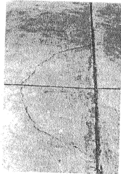
FIG. X2.4 Low-Severity Corner Break
