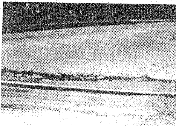
FIG. X2.40 High-Severity Railroad Crossing
