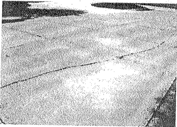
FIG. X2.7 Low-Severity Divided Slab
