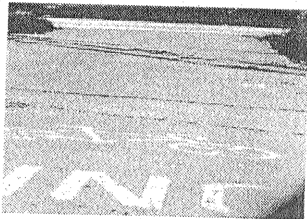
FIG. X2.39 Medium-Severity Railroad Crossing
