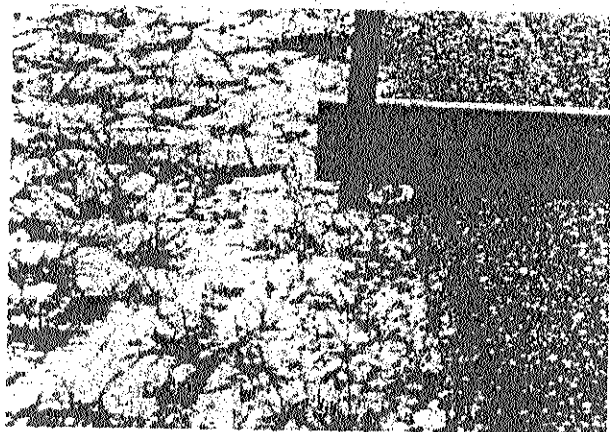
FIG. X1.25 Low-Severity Lane/Shoulder Drop-Off
