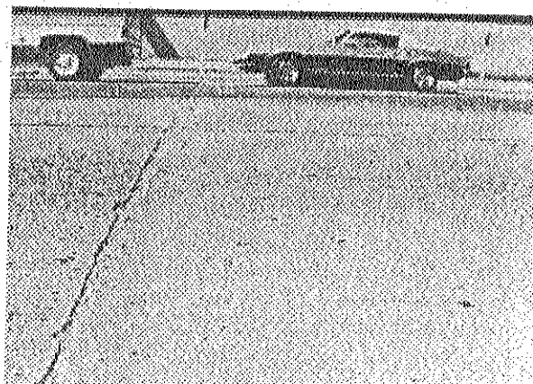
FIG. X2.48 Low-Severity Spalling, Joint
