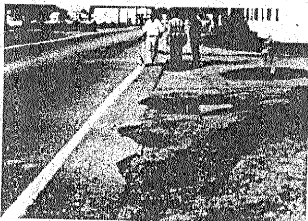
FIG. X1.21 High-Severity Edge Cracking
